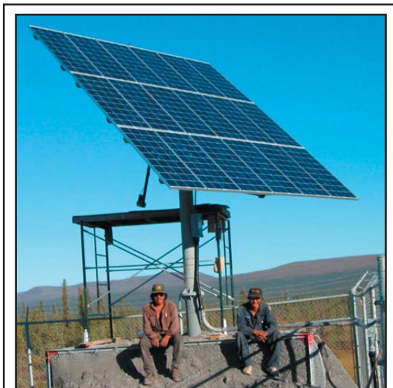
Figure 2. A state-of-the-art PV tracking system, and two local installers, near the Arctic Village washeteria.
