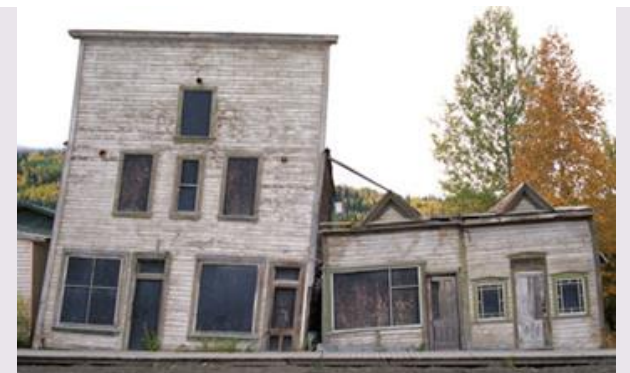
"Drunken Houses" that are falling over due to permafrost thaw
