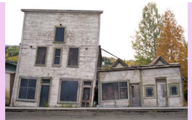
"Drunken Houses" that are falling over due to permafrost thaw
