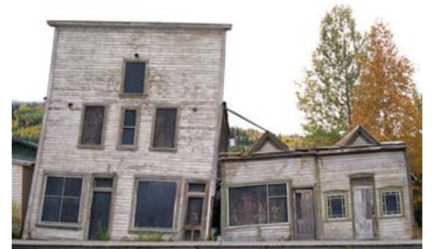
"Drunken Houses" that are falling over due to permafrost thaw
