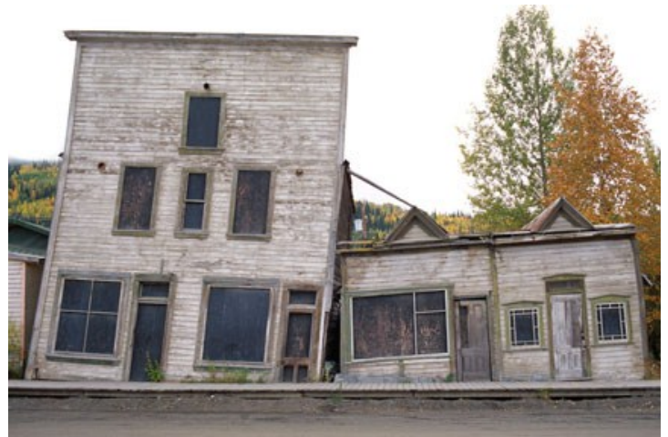
Drunken houses: buildings slump together as the permafrost beneath them thaws in Yukon, Canada. Photo: Bryan and Cherry Alexander Photography ( http://www.newint.org/features/2009/07/01/arctic-climate/ )
